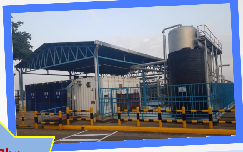
2017 Water Treatment Plant - KES 0.6bn
